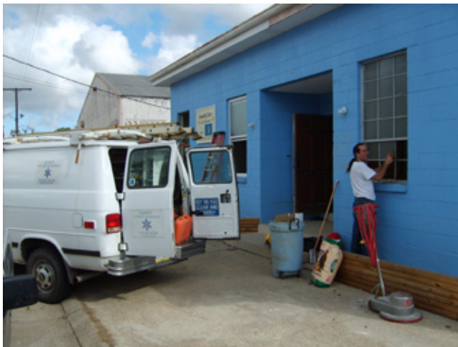
Remodeled, installed windows, offices, electricity and a bathroom, Community Center of St. Bernard Parish.
